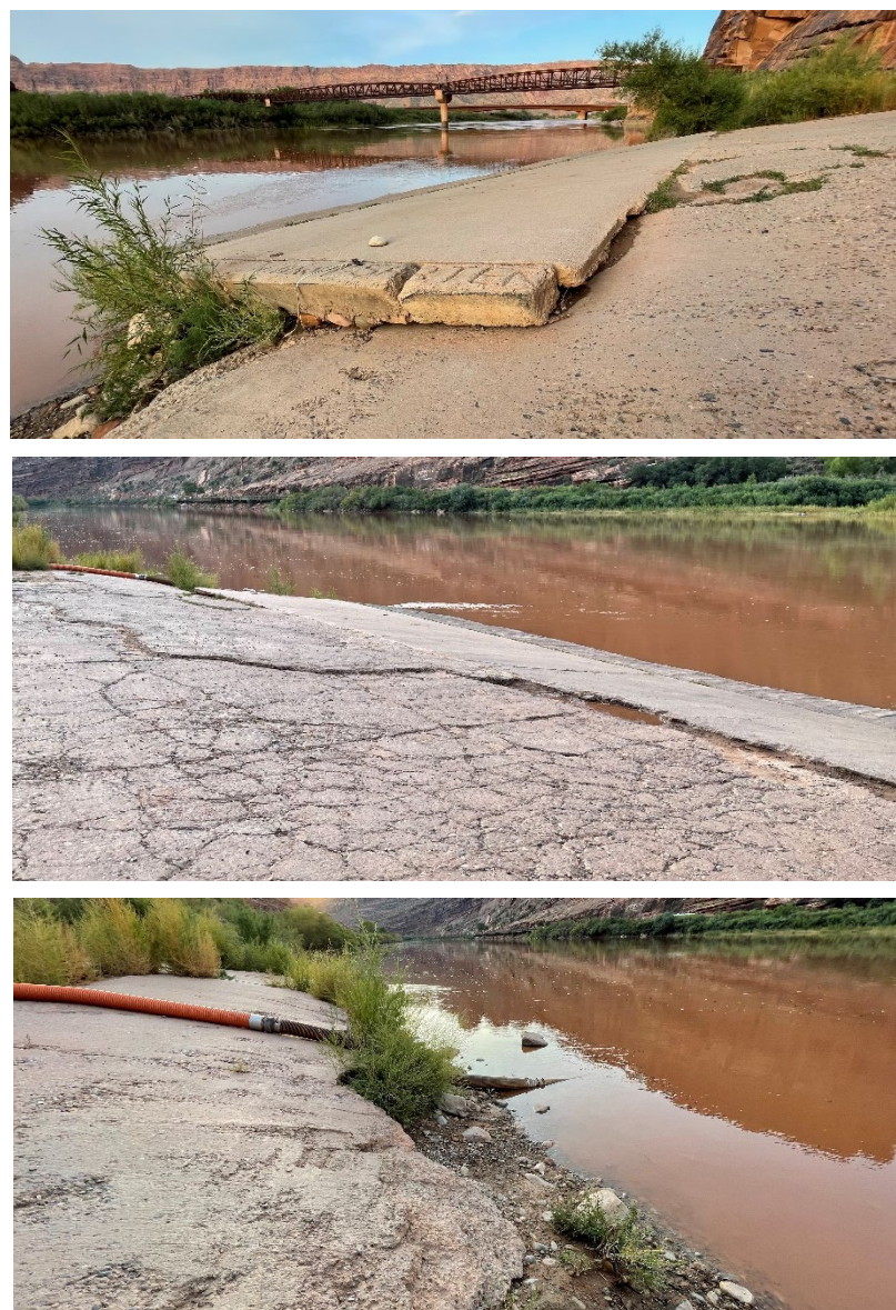
Figure 7: Photos showing poor condition of the ramp. Credit: B. Byrne
